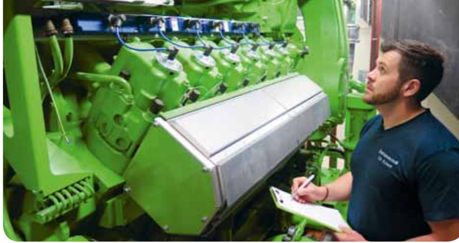
In 2015, Hermes Fulfilment commenced operation of a combined heat and power station.
